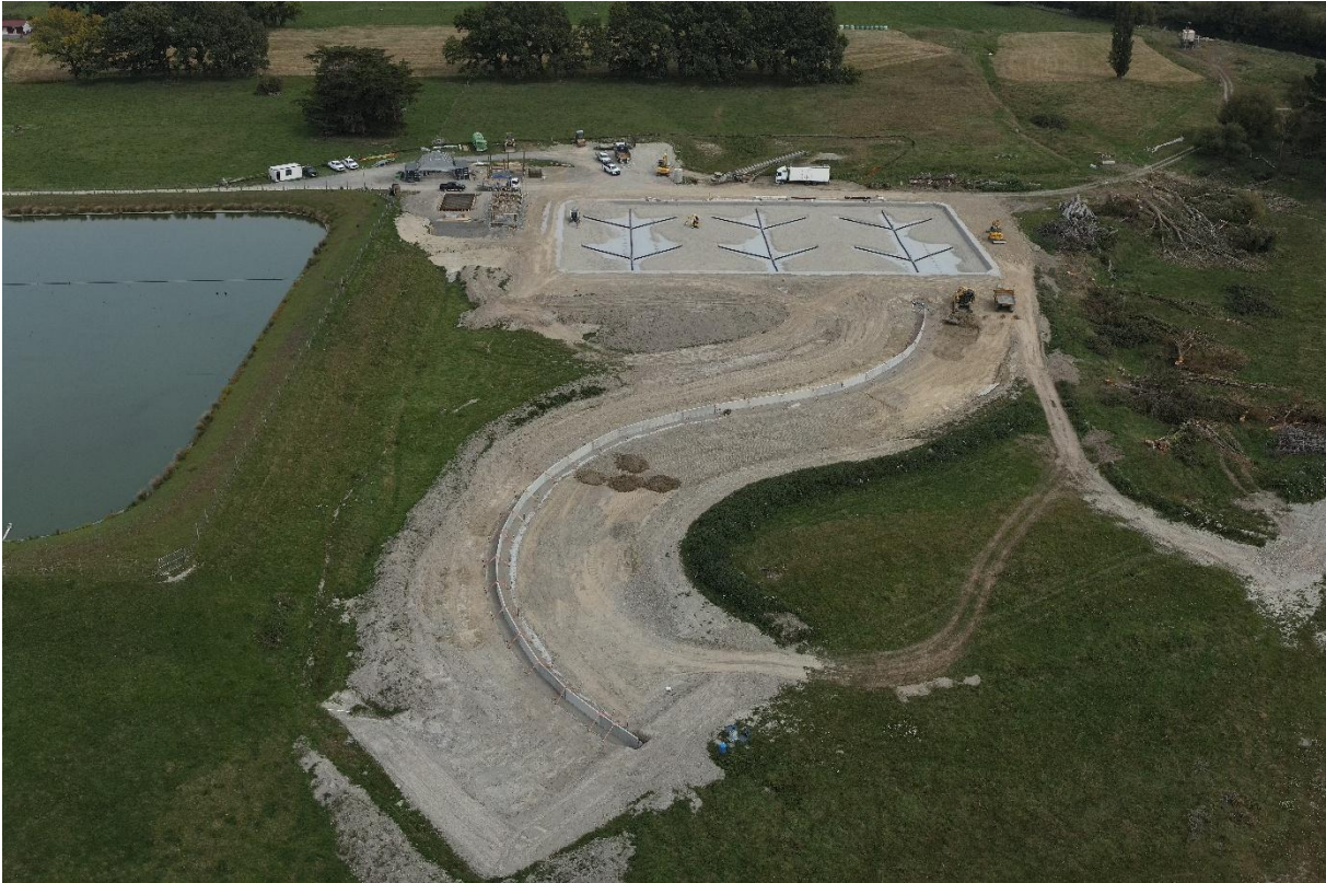
Aerial view of Pahiatua wastewater treatment plant upgrade and wetlands under construction.
