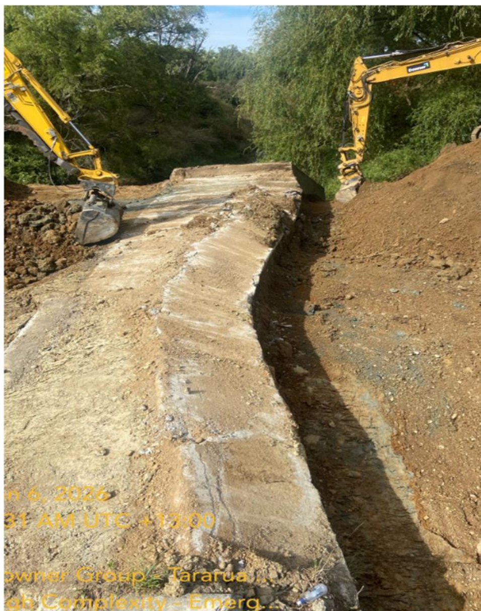
Daylighting the Old Otanga (culvert with the collapsed section in the middle)
