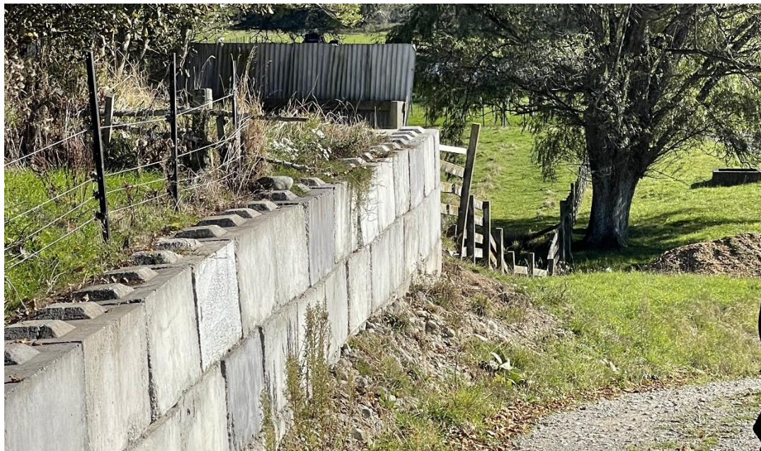
Pahiatua Water Treatment Plant fencing issue
