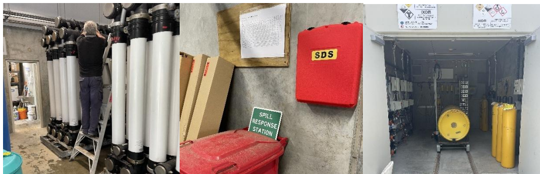
Pahiatua Water Treatment Plant
