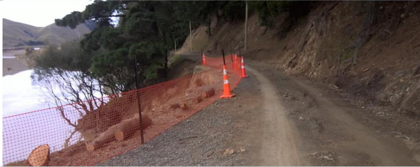
February 2023 – Access to Owāhanga Station was near severed in Cyclone Gabrielle. The river had scoured into the road, leaving 4m of width between a steep upslope and edge of dropout.
